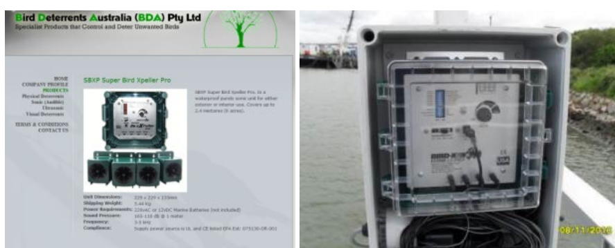
Figure 6 Audible bird deterrent installed on pontoon
