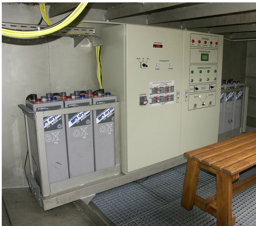
Figure 3 - Installation of Gel batteries in a signalling float
