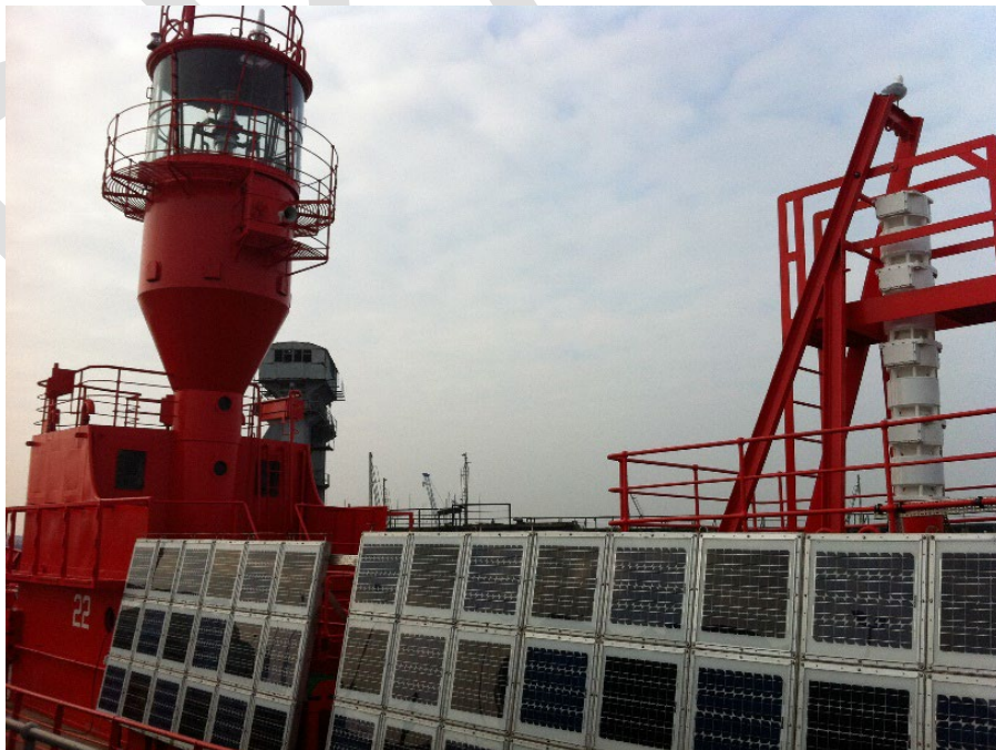
Figure 22 An example of a solar array on a lightvessel
