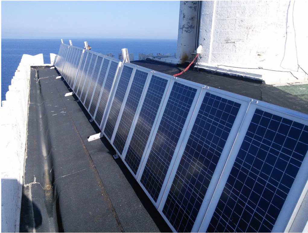
Figure 21 Photo of a solar array on La Giraglia lighthouse, Corsica
