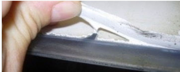
Figure 33 Examples of sealant failure.
