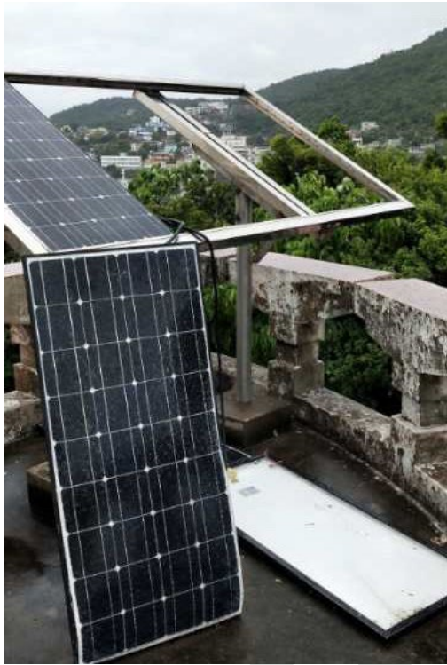
Figure 23 Example from China of damaged solar modules following a super typhoon
