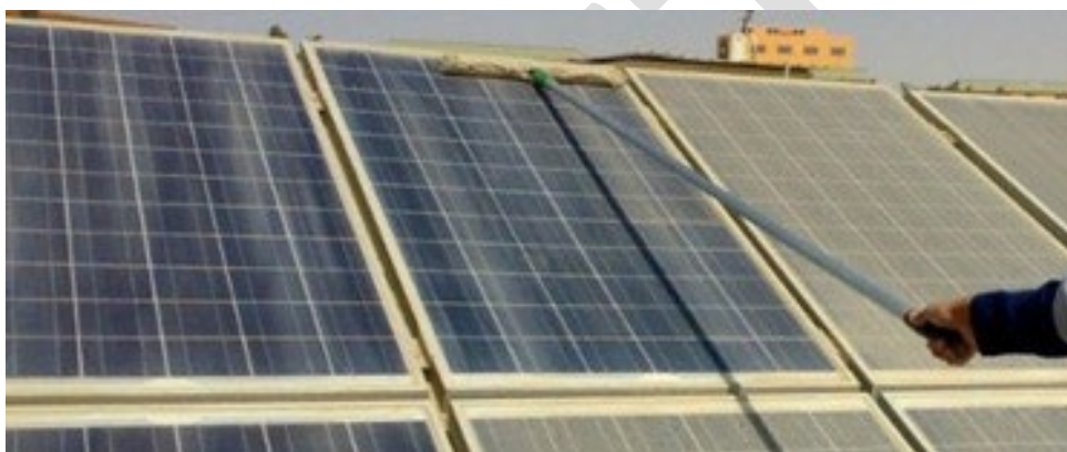
Figure 18 An example of heavy dust deposit
