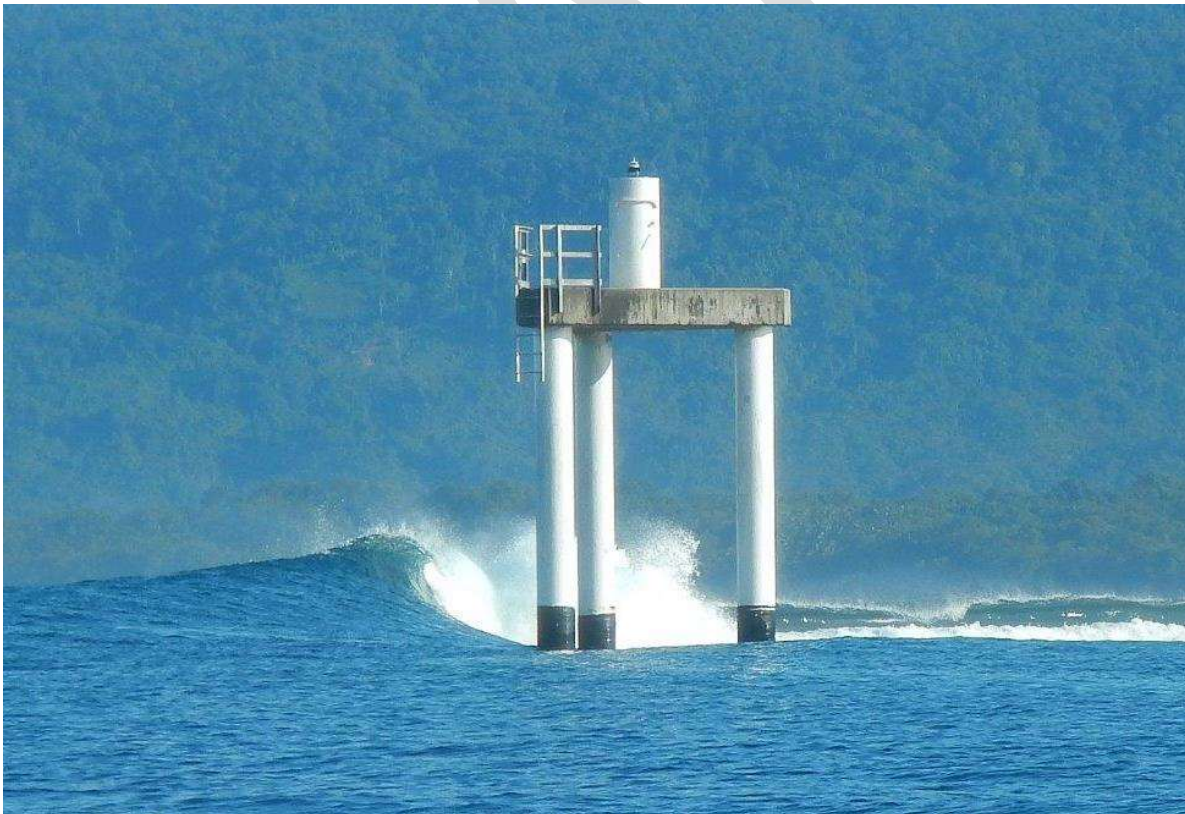
Figure 2 Example of multi-steel piled, concrete light platform with GRP light tower, access ladder and tape wrapped piles within the splash zone
